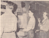
Richard Brown, EM2, Fred Flores, PN, Thomas Green PN Paralleling additional turbo generators prior to flight operations.
