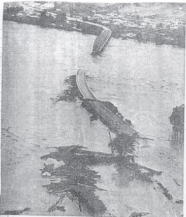
The rampaging Eel River literally ripped the Paul Mudgett Memorial Bridge asunder. Rio Dell is in the background. The Eel River sawmills were formerly located at the lower left. Note the debris remaining where houses smashed against the left side of the span.
