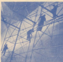
High along the hull of the Bennington, members of the Joiner & Shipwright Shop remove one of the last remaining bays of pipe staging just before the ship's launching.
